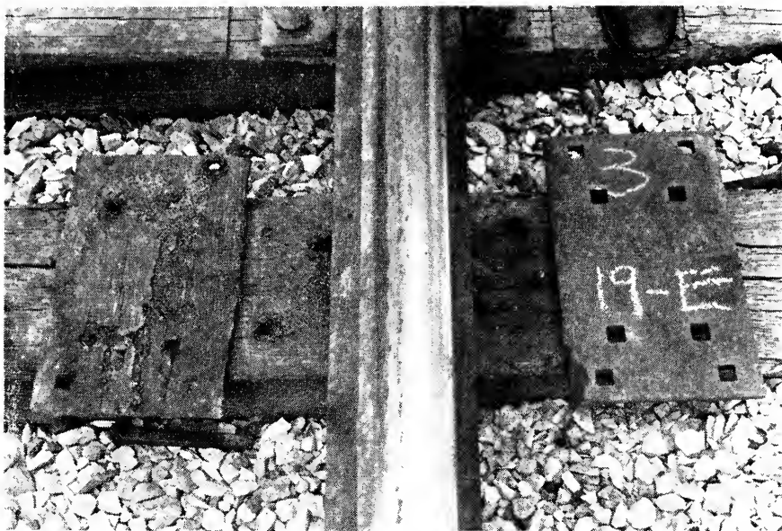
FIG. 16. Section 3, 13-in Fiber-Rubber Tie Pad. Abraded Surfaces. Coated. After 25-months' Service in the Inner Rail of the Long 4-1/2° Curve.
